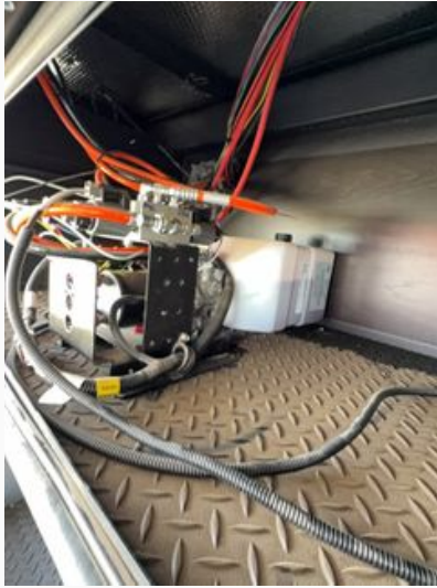
overview of pump
