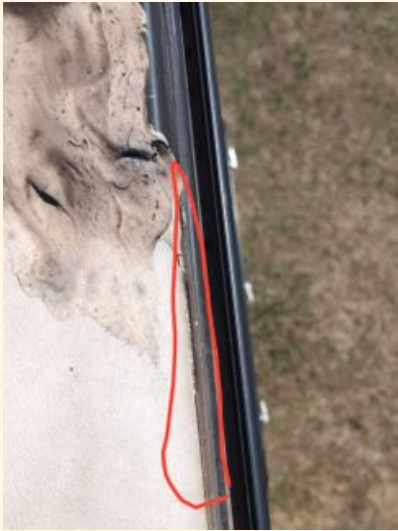
Front Curbside Rail Trim Cracks in Sealant
