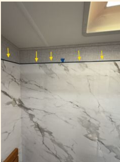
Gaps in sealant
