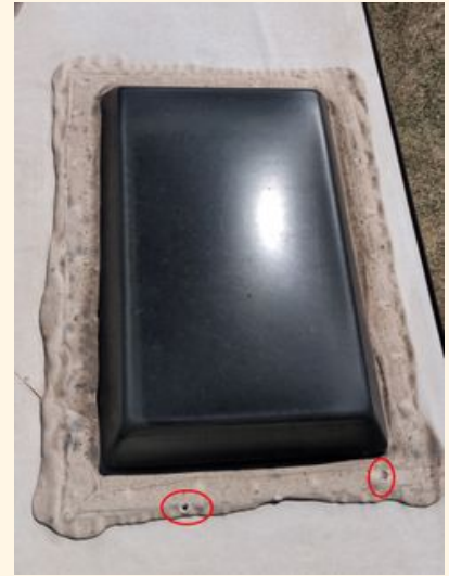
Skylight Holes in sealant
