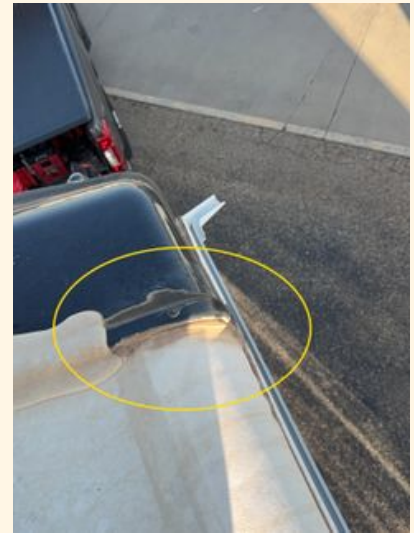
Location where sealant is failing
