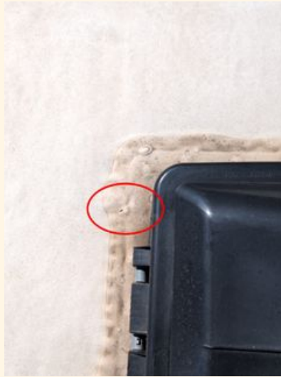
Ceiling Vent Hole in Sealant
