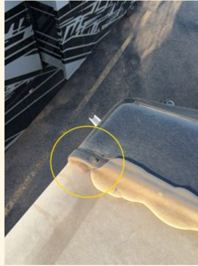
Zoomed out Location of failed sealant
