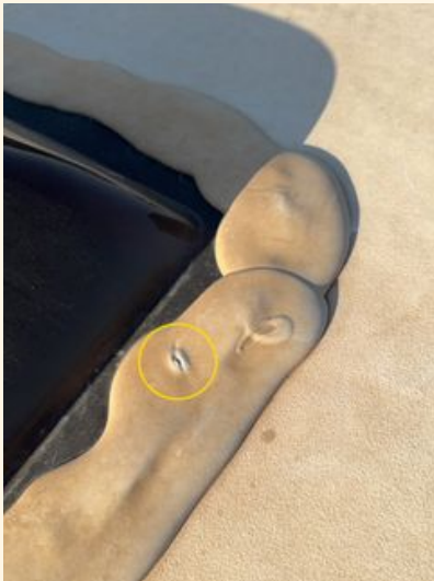
skylight sealant air bubble
