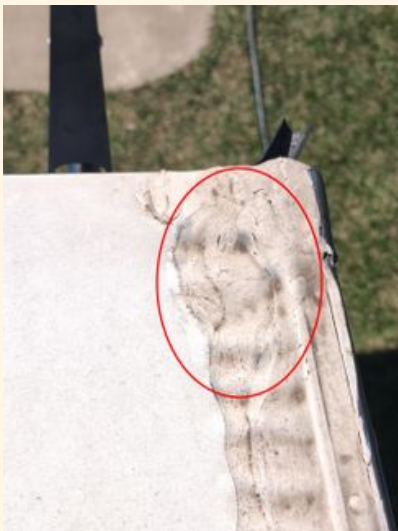
Curbside Rear Cap Holes in sealant
