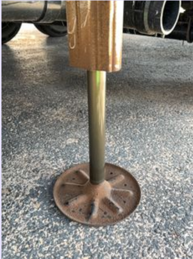
seal leak, this is why actuator is so dirty because the seal is leaking
