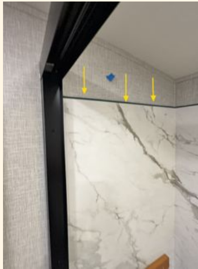
Gaps in sealant
